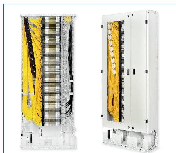
Front Access Cabinet (without and with doors) | Photos CRR2826, CRR2741
